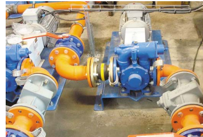
Heating Oil transfer
