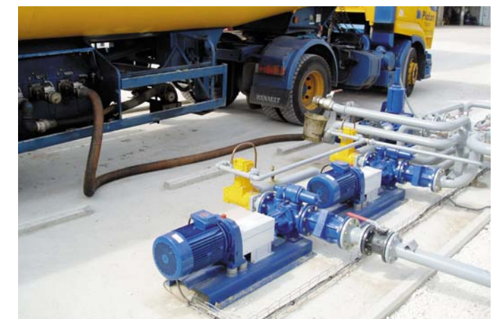
Truck loading (Heating Oil)
